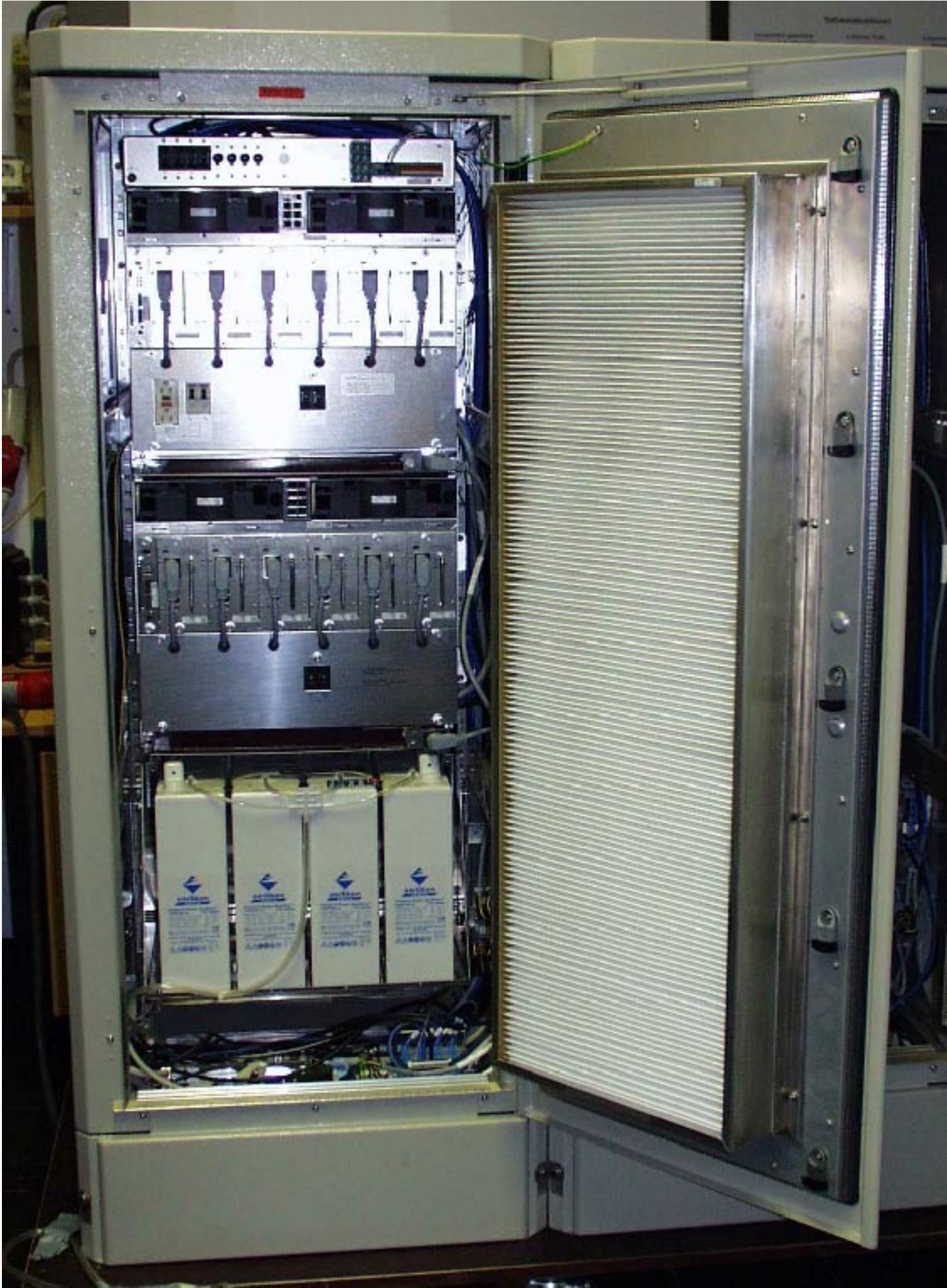
BS-241U Service shelter - Front door open
