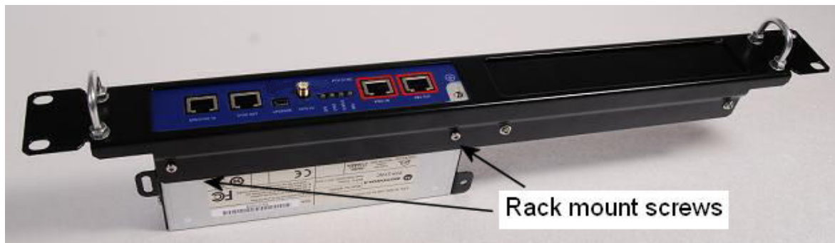
Figure 96 PTP-SYNC mounted in a rack
