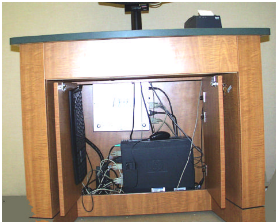
Typical In-Desk Setup (Door Open)
