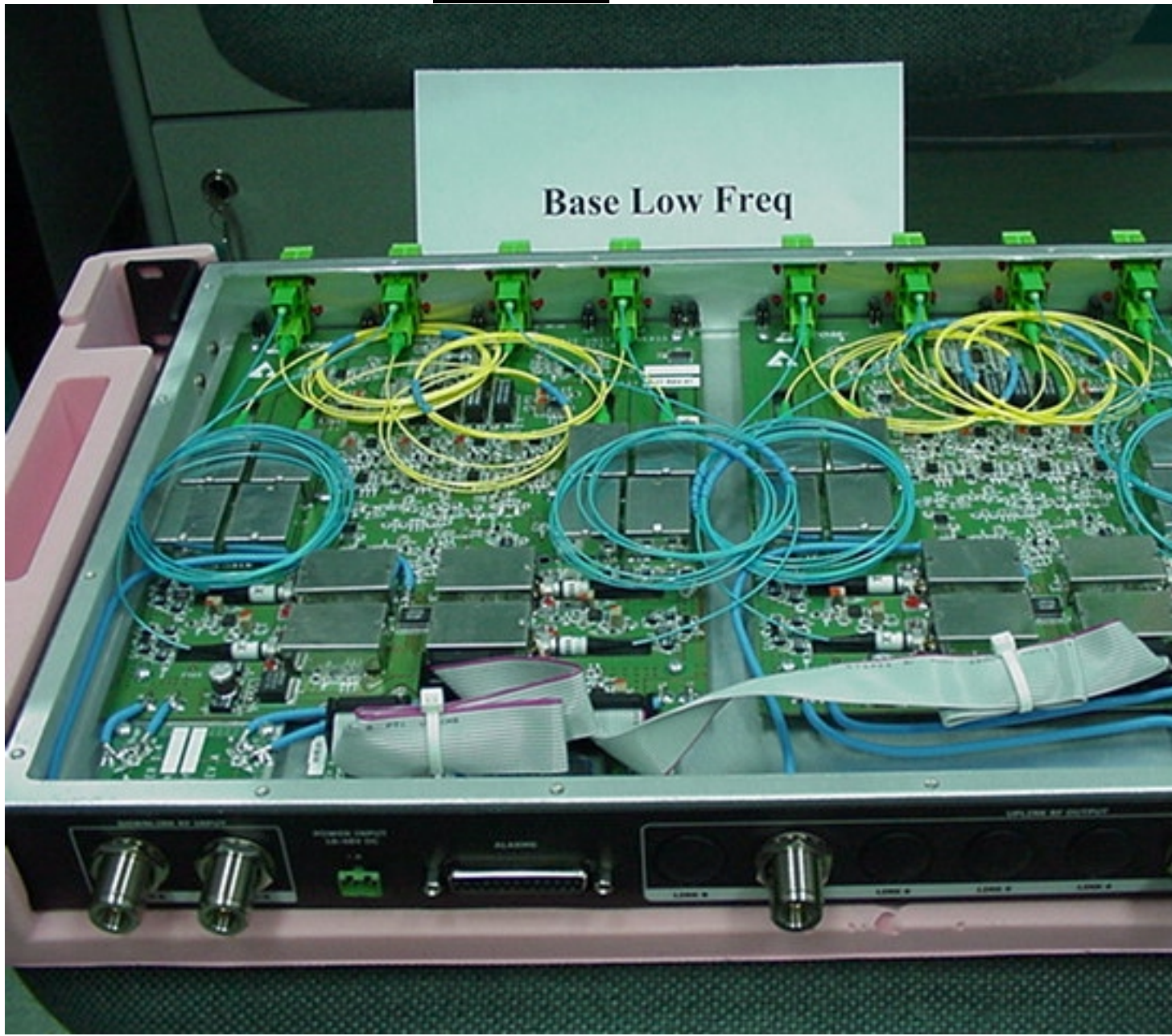
BASE STATION LOW FREQUENCY
