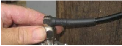
Figure 7: Verify connection of RF cable
