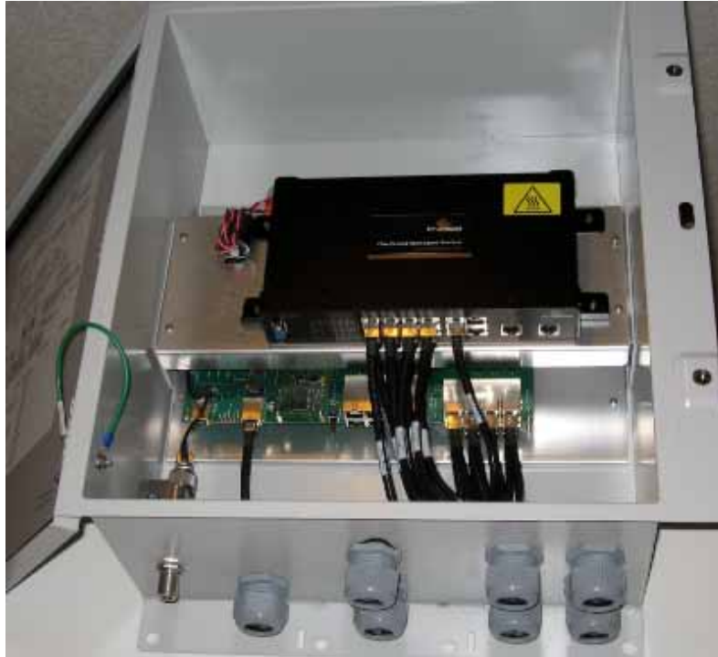
Figure 40 CMM4 (Cabinet with switch)
