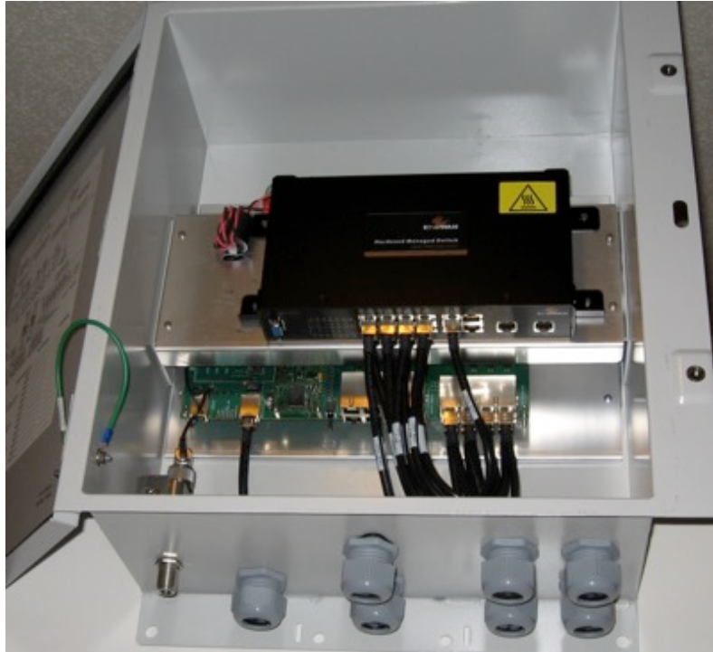
Figure 17 CMM4 (Cabinet with switch)
