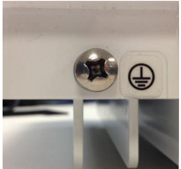
Figure 8: Single-Hole Ground Hole (M6)
