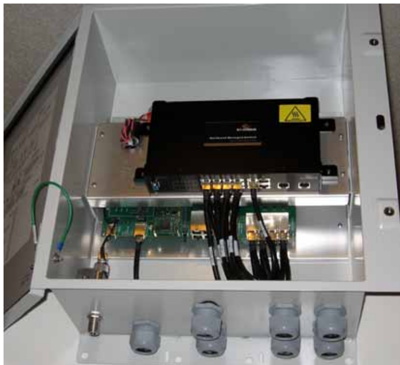
Figure 36 CMM4 (Cabinet with switch)
