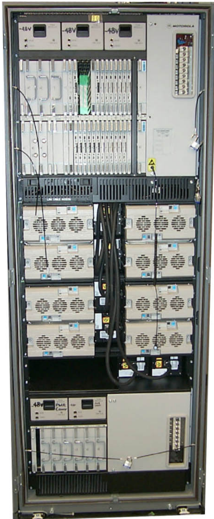
IHET5AW1 -48V SC4812T 800 MHz Front View Door Open
