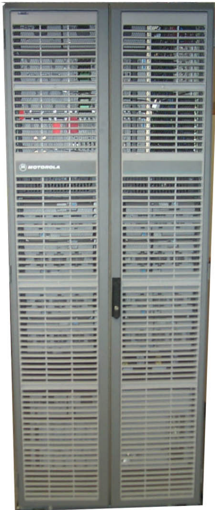
IRET5AW1 -48V SC4812T 800 MHz Front View Door Closed
