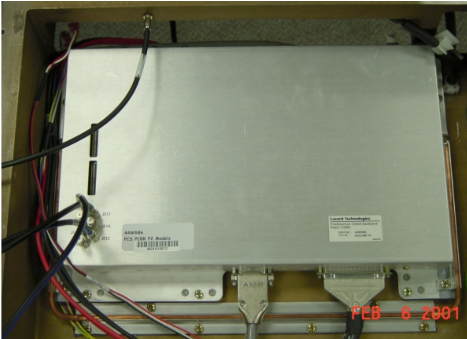
Photograph 1: PCBR Installed in RFU Cabinet
