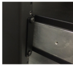
Figure 1b: Rack installation
