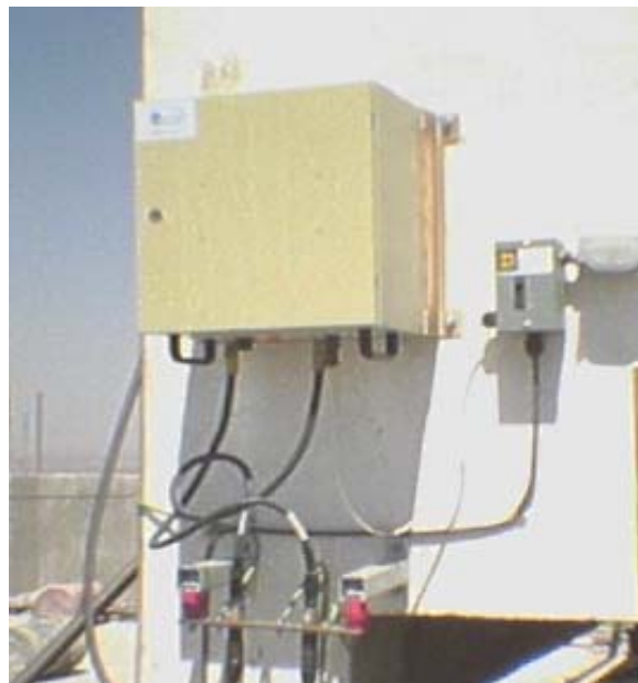
Figure 45: CDMA Repeater – Typical Outdoor Installation
