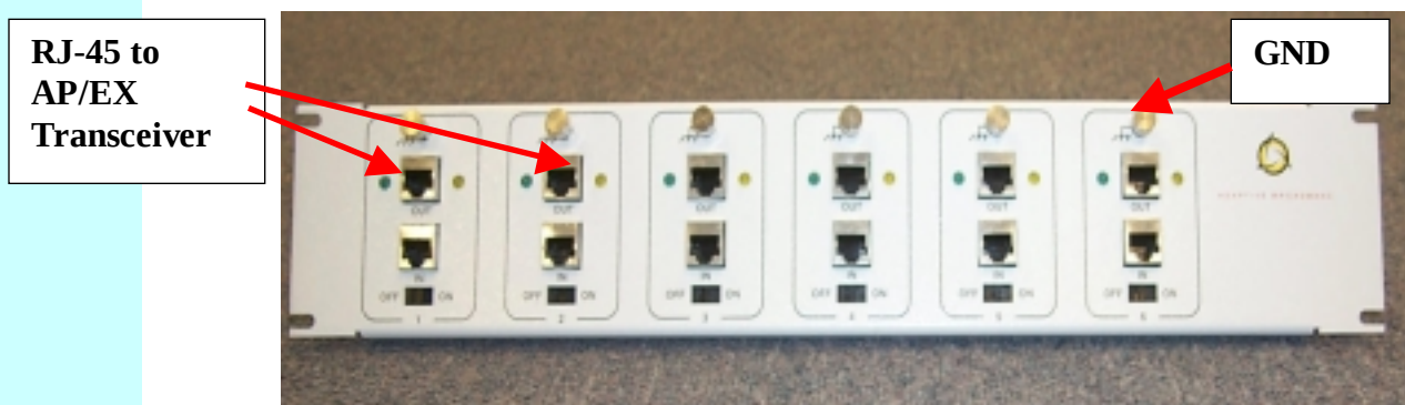
Figure 6-14 Access Panel showing Connections to AP/EX
