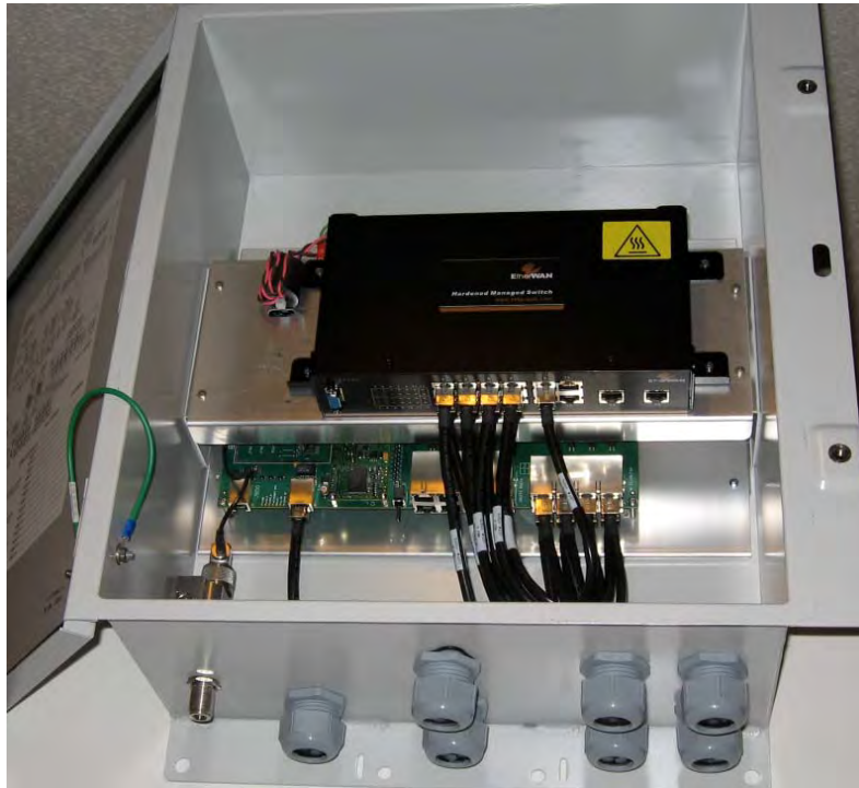
Figure 26 CMM4 (Cabinet with switch)
