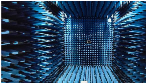
Figure 2: Geometry of Anechoic Chamber for Radiation patterns.
