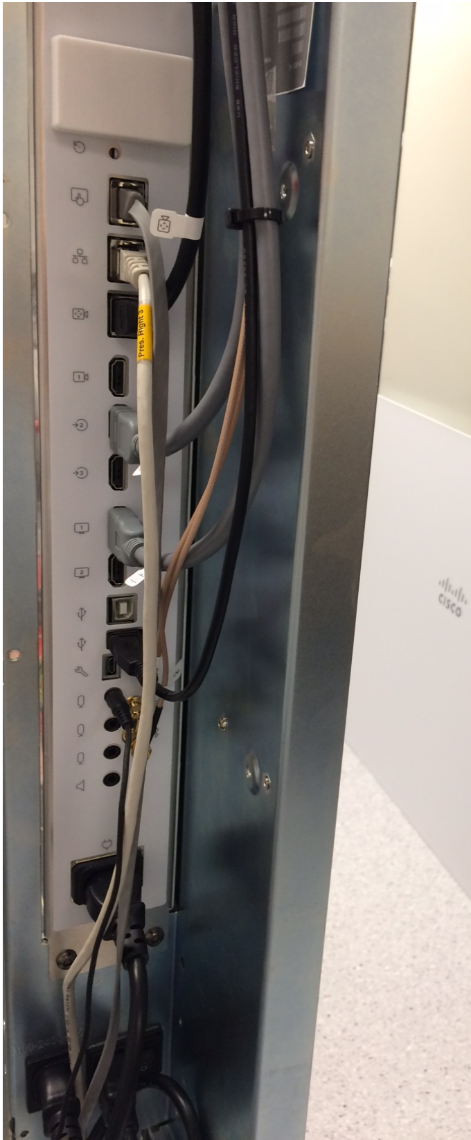
I/O panel close up
