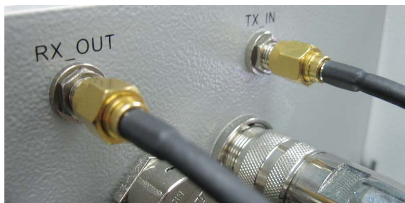
SMA Coaxial Cable Inter-connection on Single-band Enclosure
