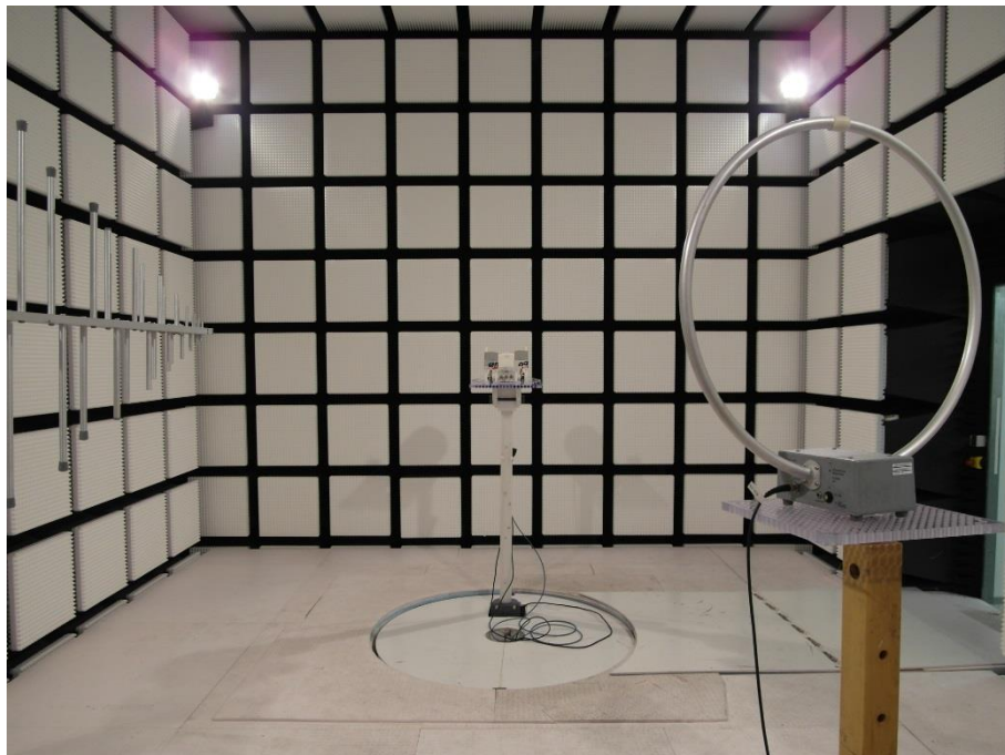
Photo 18 - Measurement Chamber A – SPA 5600/40/14/0/V_2:
