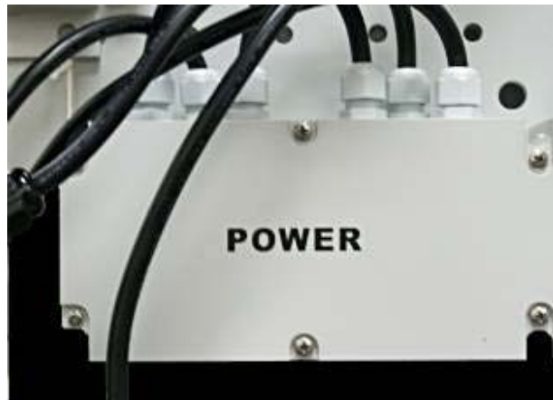
Figure 35 AC Power Junction Box
