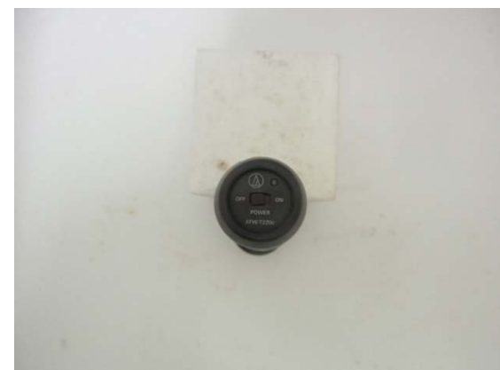
Photograph A6: Bottom
