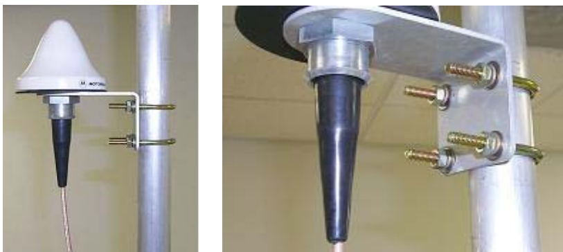
Figure 29 GPS antenna mounting
