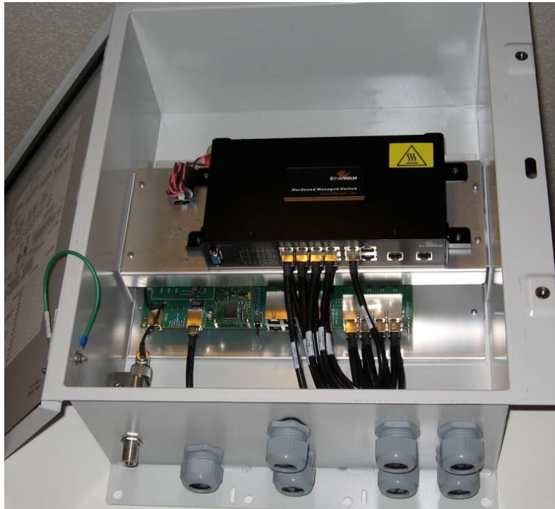
Figure 26 CMM4 (Cabinet with switch)
