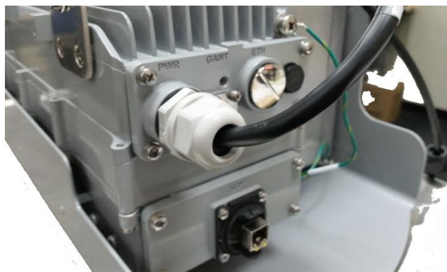
Figure 31: Power cable attached to AirHarmony-1000D
