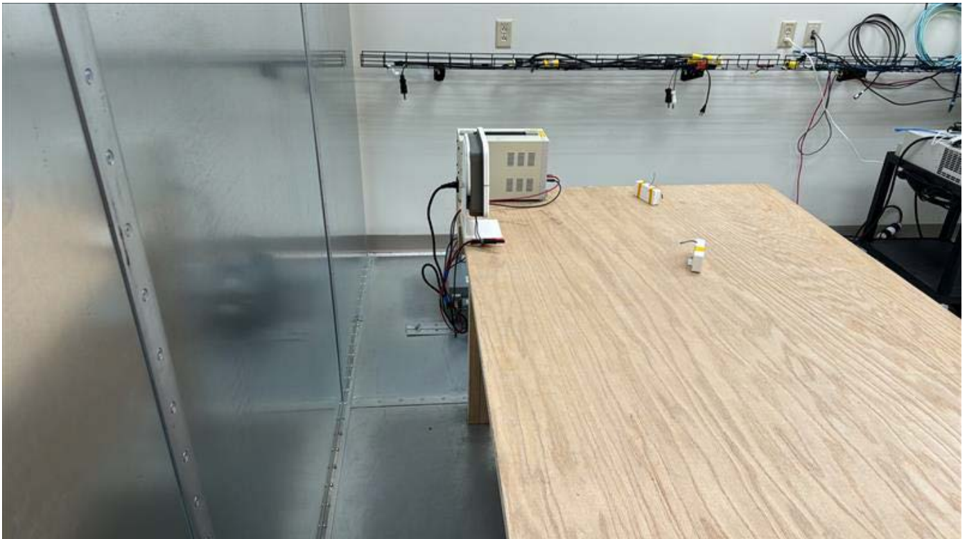
DC POWER MODE AC Line Side
