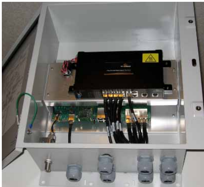
Figure 40 CMM4 (Cabinet with switch)
