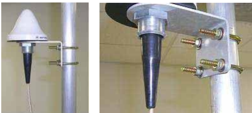
Figure 43 GPS antenna mounting
