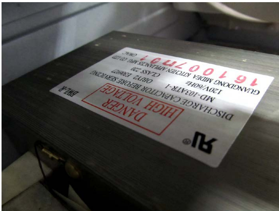
High-voltage Transformer view
