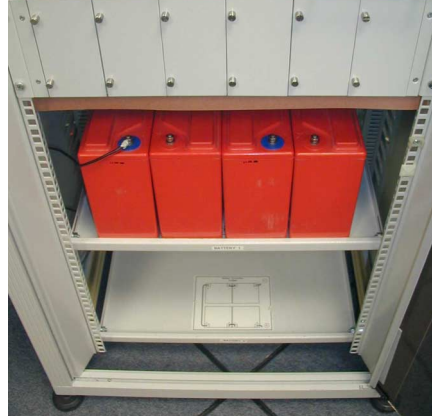
Figure 7-6: Cabinet battery area
