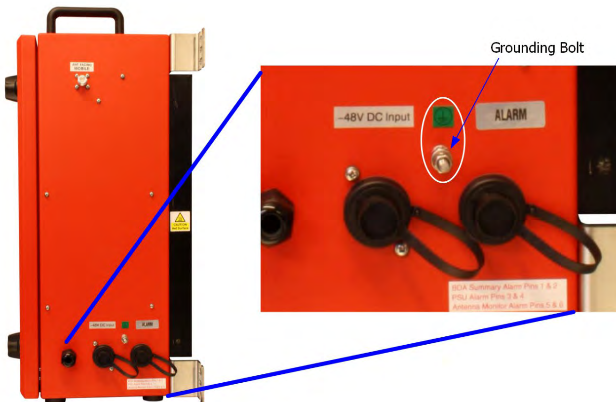
Figure 4-9: Grounding the BSF-3604
